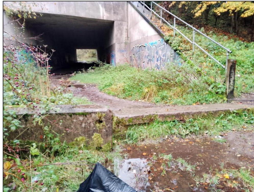
Photograph 1B Route through subway is unlit, muddy and uneven (but can be seen that the route is regularly used).
